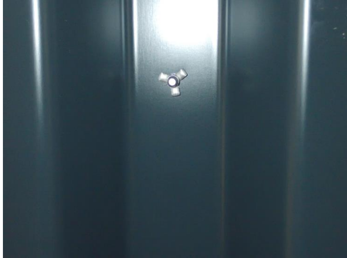
Photo 4 Detail of a rivet on the backside of the trapezoidal sheet.
